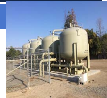
1,2,3-TCP Wellhead Treatment
