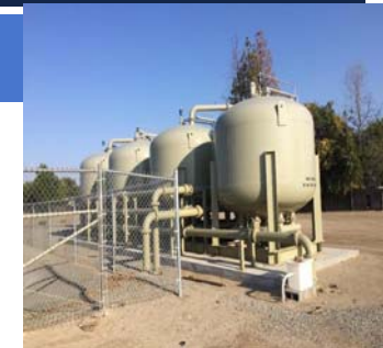
1,2,3-TCP Wellhead Treatment
