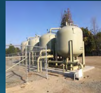
1,2,3-TCP Wellhead Treatment
