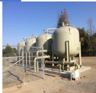
1,2,3-TCP Wellhead Treatment
